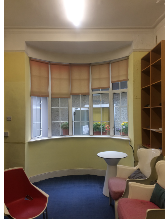
Existing uPVC windows to be replaced and bay window to be rebuilt up to parapet level as advised in the Timber and Damp Building Investigation Report that forms part of this application. New blinds, Thermal upgrade works to external walls - Note existing coving
