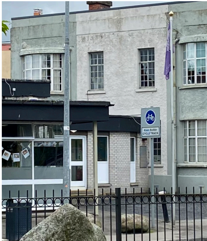
Existing opening to protected structure to be made good where 1970's building will be demolished.
