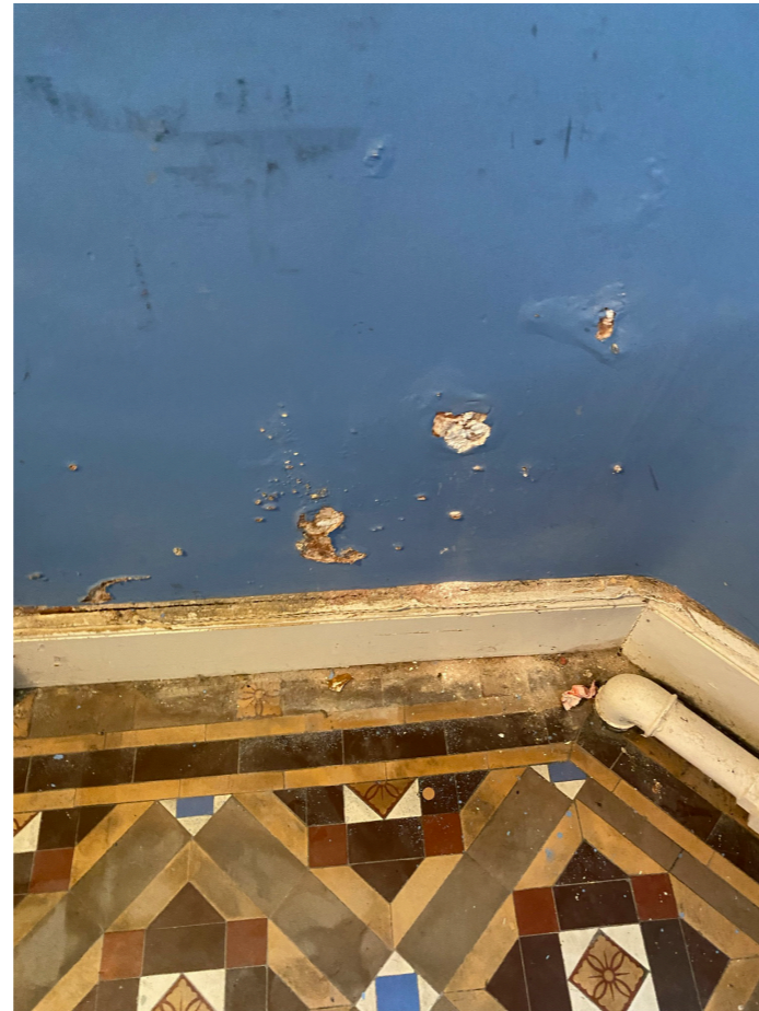
Damp issues to be investigated and resolved prior to thermal upgrade works, Refer to Timber and Damp Building Investigation Report
